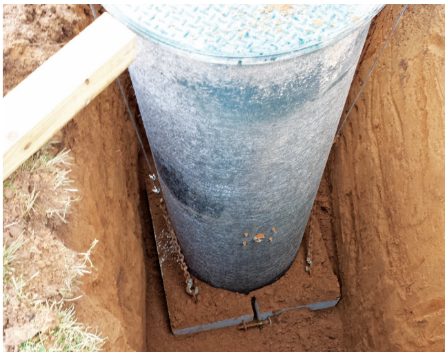
Collection System Grinder Pump Basin
