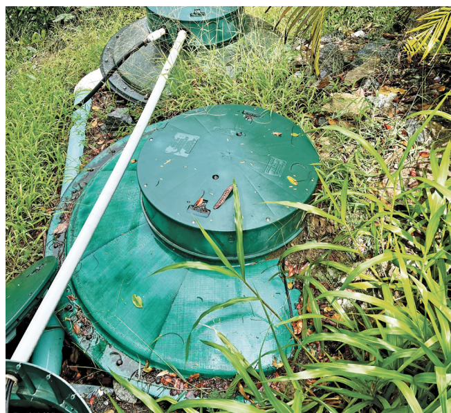
Aerobic Treatment Unit (ATU)
