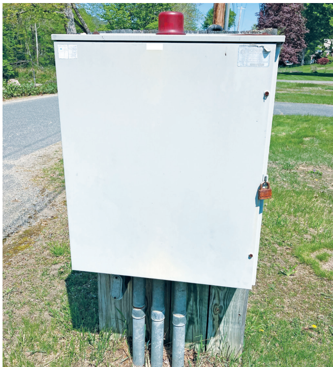
OWTS Control Panel
