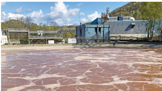
Activated Sludge Aeration Tank
