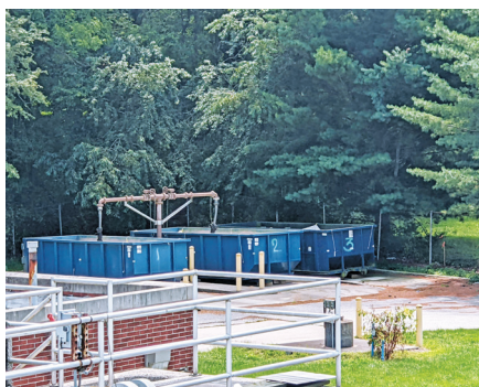
Dewatered Sludge Bagging System
