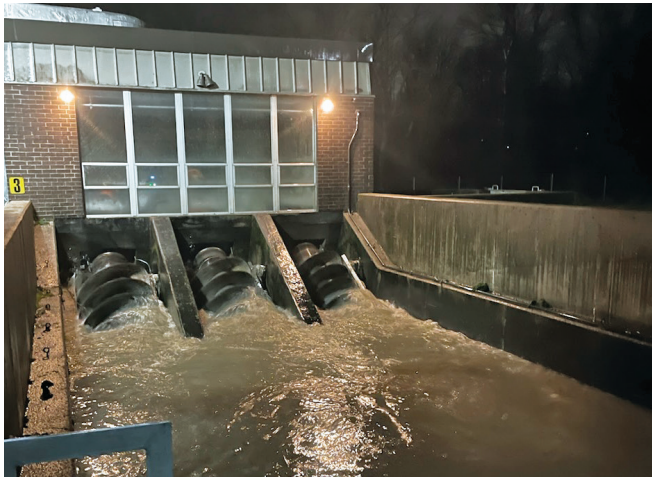
Influent Screw Conveyors
