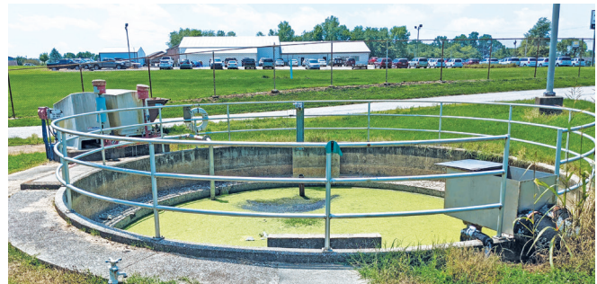
Aerobic Sludge Thickener
