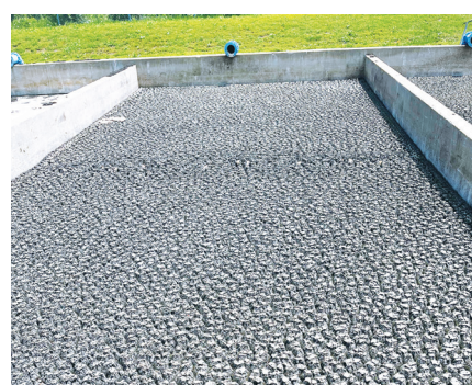
Sludge Drying Bed
