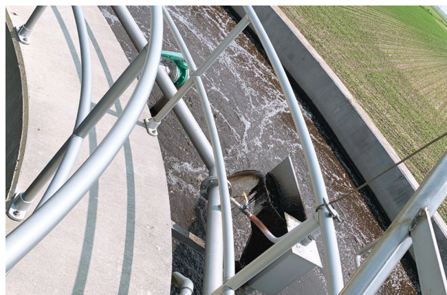
Extended Aeration Tank
