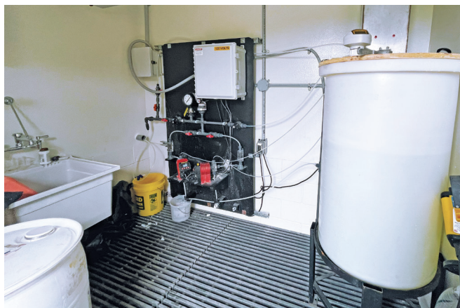
Liquid Chlorine Disinfection
