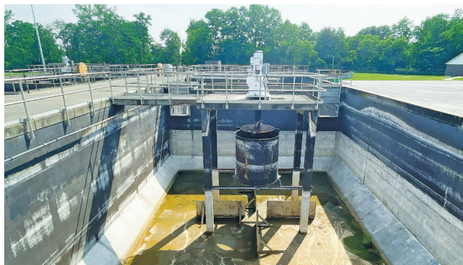
SBR Reactor - Empty
