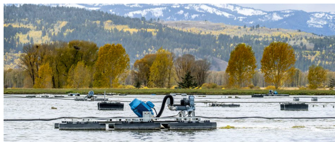
Figure 5. Aerated Lagoon. Figure 2. Midwest Assistance Program. (2021). Intro into Wastewater and Lagoon O&M. [PowerPoint Presentation]
